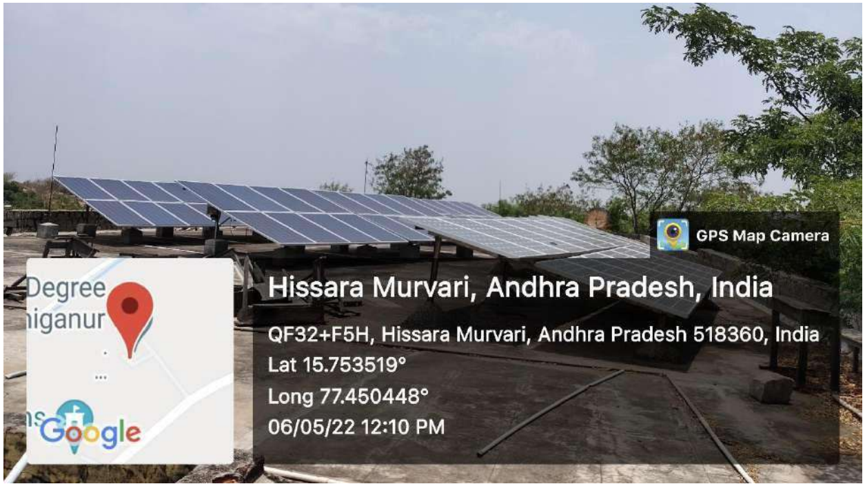
Solar Panels on the roof of Old Building
