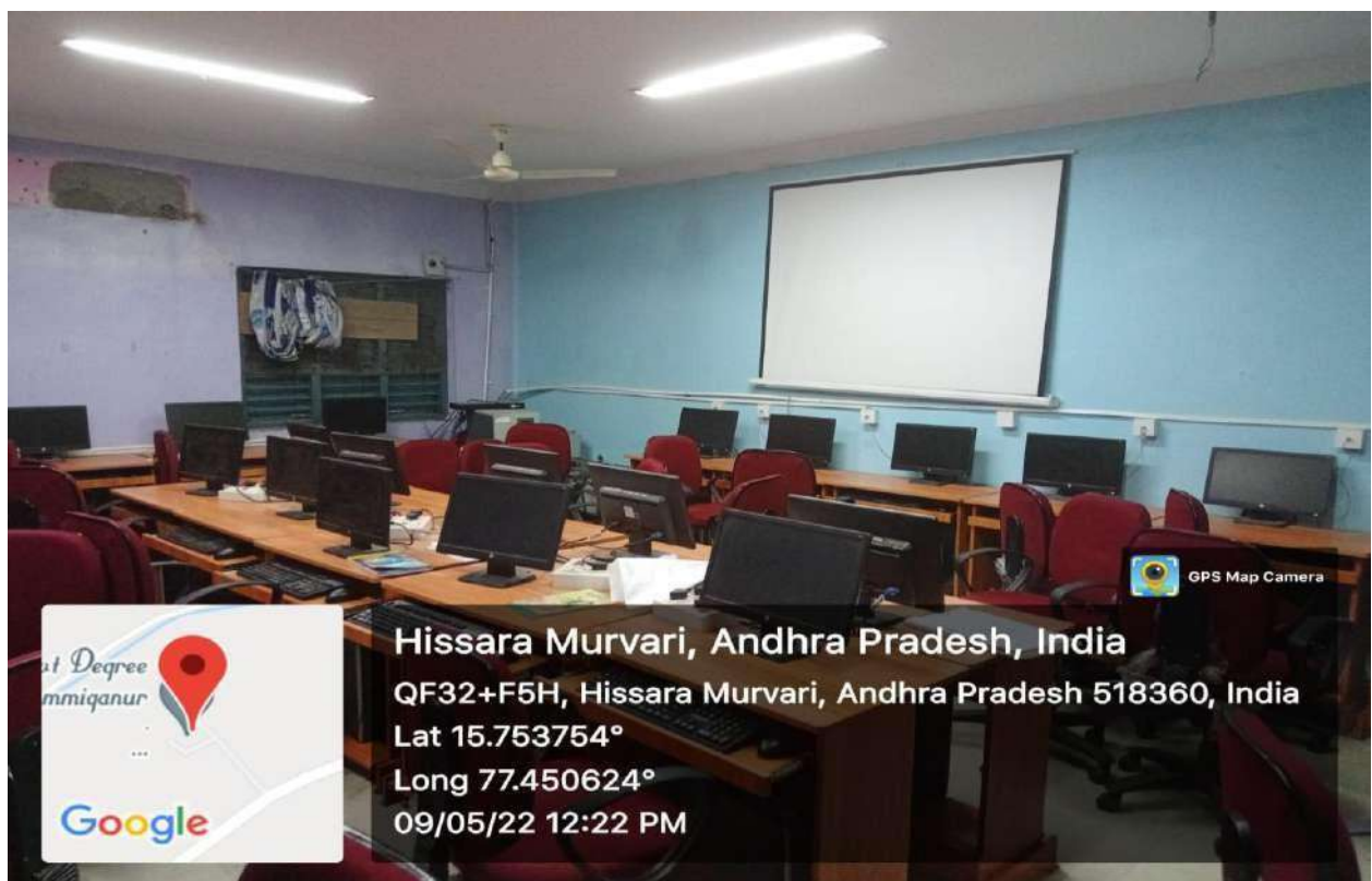
Usage of LED lights to conserve electricity in ELL Lab
